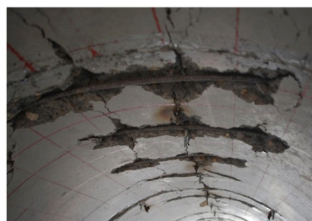
b. local damage effect of rear face
