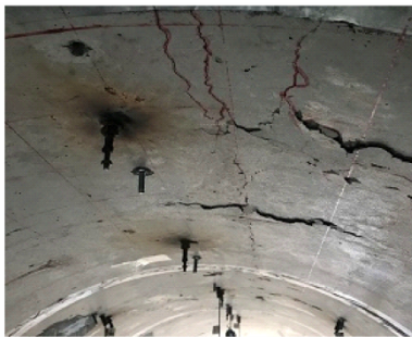
b. local damage effect of rear face
