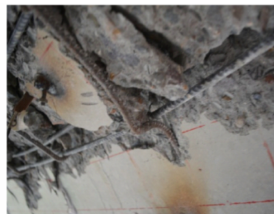
b. local damage effect of rear face
